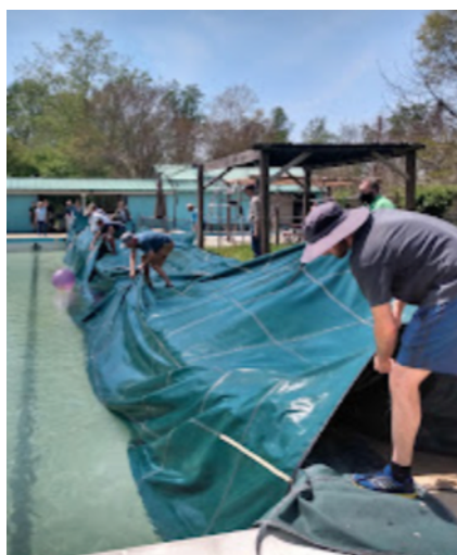
Many volunteers worked to uncover the pool at a work day in April. Photos: Paola Addamiano-Carts.
